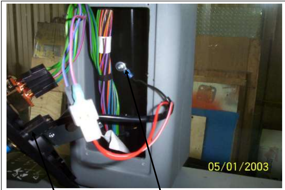
A/C switch mounted on switch panel
