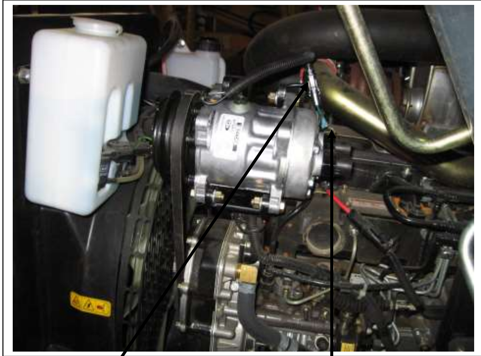
Compressor clutch wire attached to binary switch.
