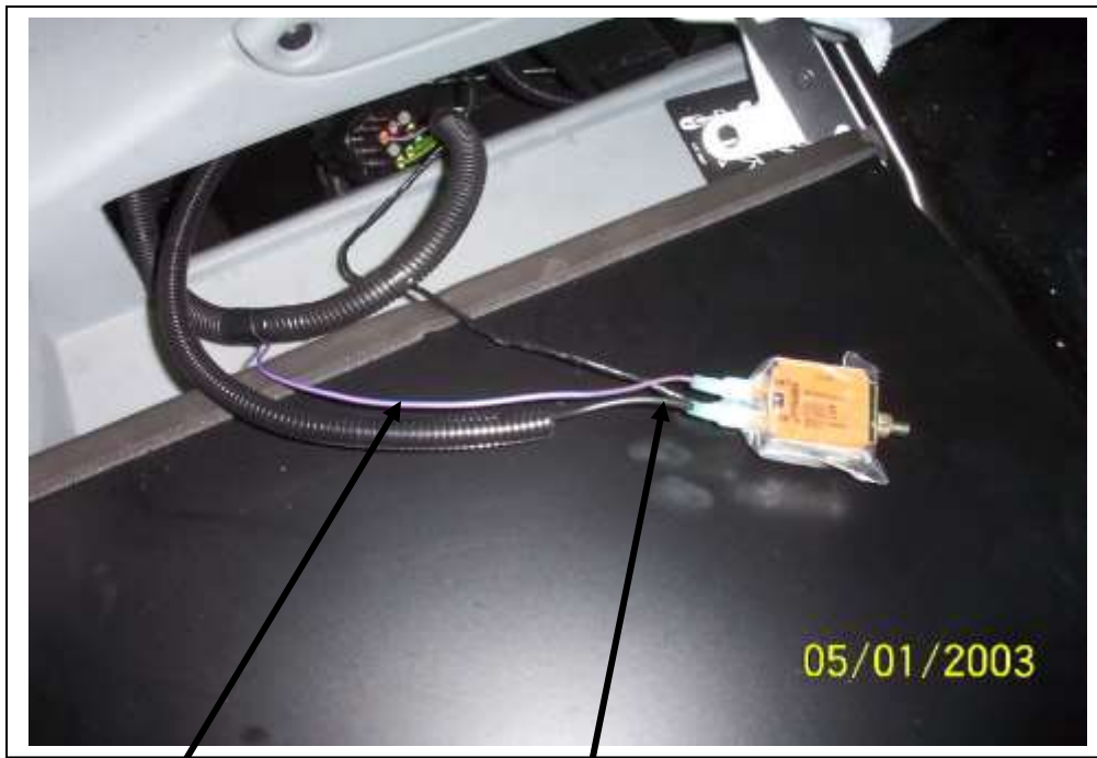
Wire from A/C switch on control panel.
