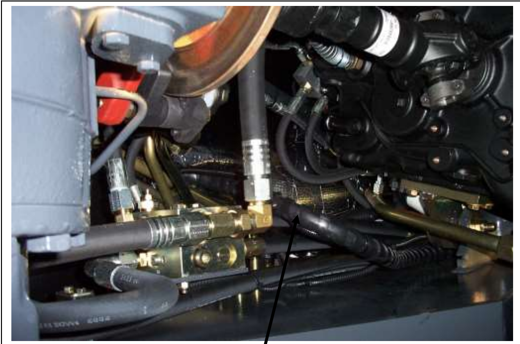
1/2" hose running up and over the rear axle and heading to the right side of the machine to the AC fittings at the heat/AC box.
